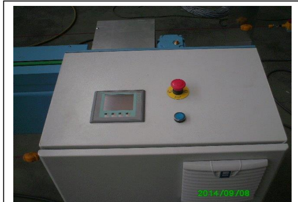
Electric cabinet with Touch Panel
